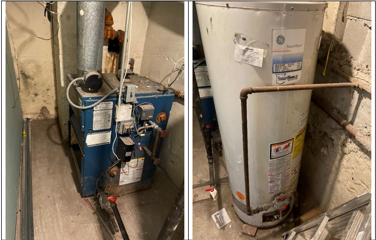
(Boiler and Water Heater)
